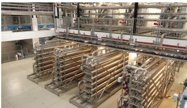
New makeup water preparation system
